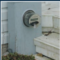
Deck Staircase Built Around Pedestal Meter Socket (Meter Cannot be Removed)
