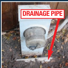
Looking Down on Meter Pedestal Drainage Pipe in Front of Pedestal (Meter Cannot be Removed)
