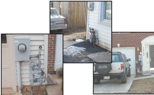
Example of meter protection violations
