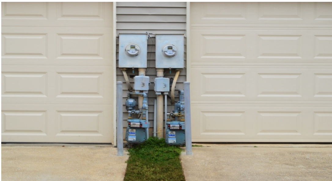
This is a representative photo of gas meters and bollards.
