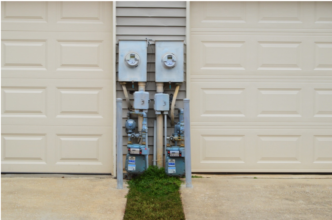
This is a representative photo of gas meters and bollards.
